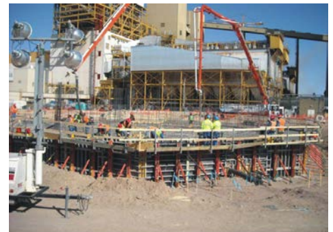
Coronado Emissions Control Project
