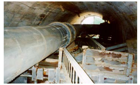
Bear Valley Hydroelectric Plant Penstock
