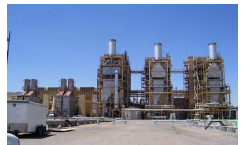
Newman Generating Station
